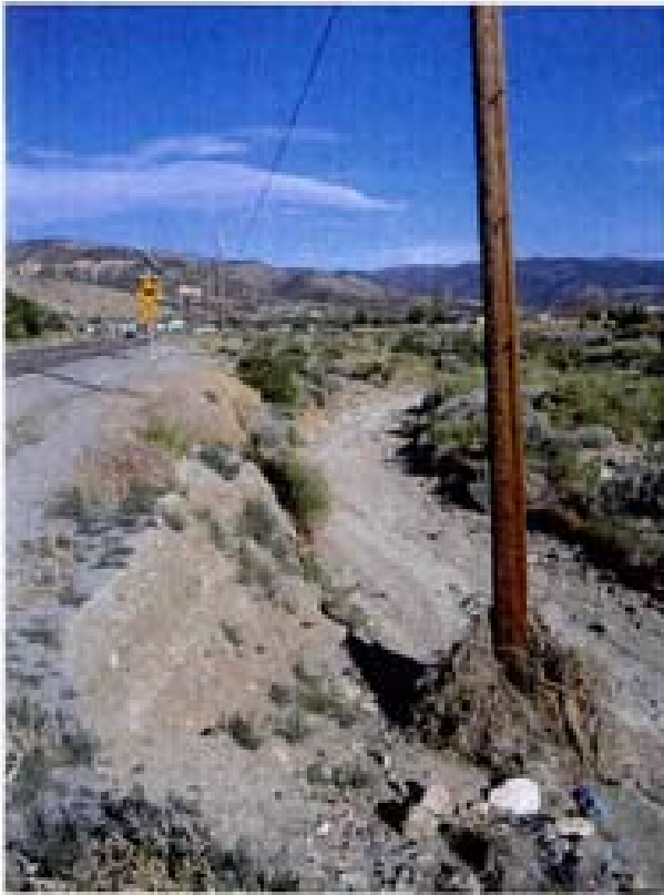
Erosion along Bailey Canyon Creek adjacent to Undercutting along a private parcel
