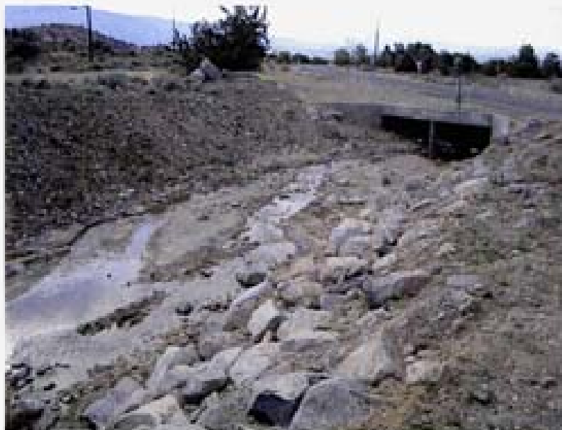
Channel configuration and sediment accumulation in the RCB culvert under Toll Road near Ravazza Road.
