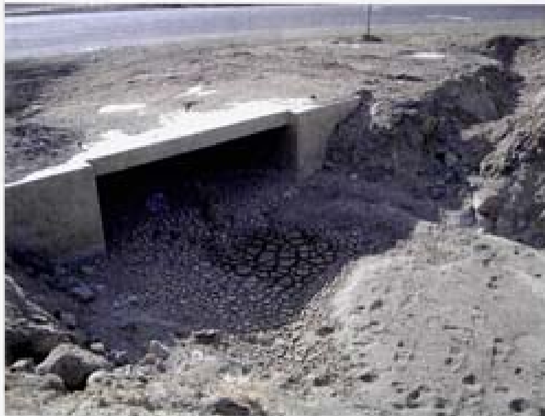
Sediment accumulation in the 12-foot by 4-foot RCB culvert under Toll Road near the intersection with Geiger Grade.
